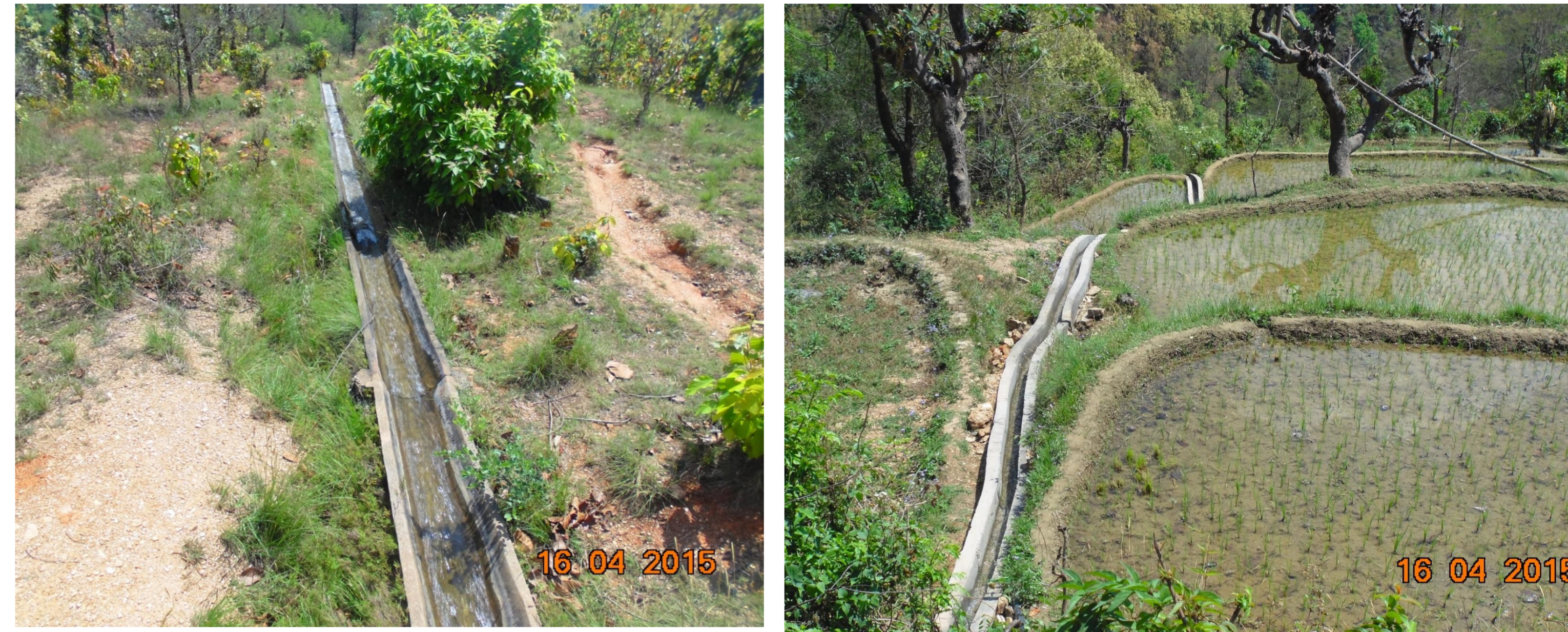
Efficient section canal lining on the farm level in remote hills of Nepal.
