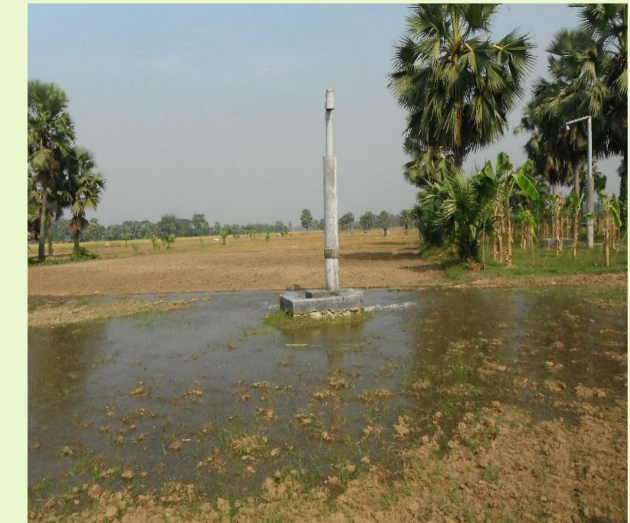
Outlet from buried pipe system and air-vent standpipe
