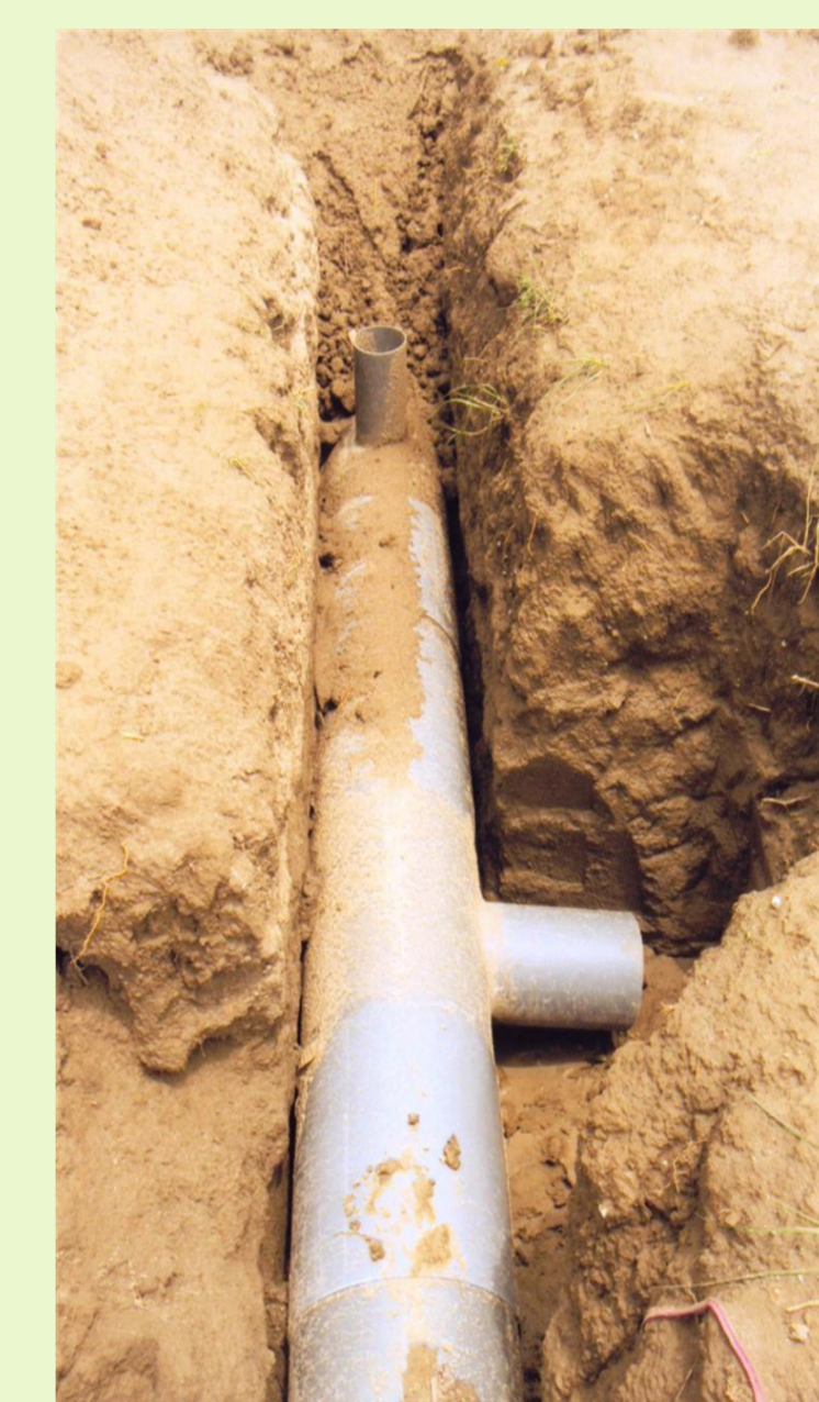
uPVC Buried pipe
