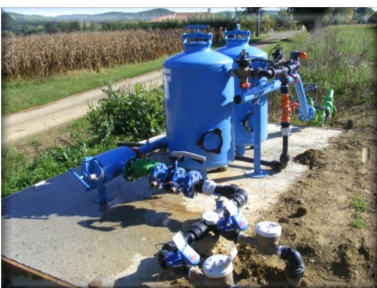
Figure 3 : station de filtration
