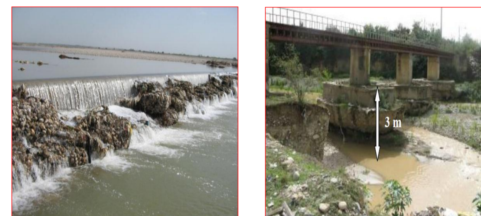
Figure(6): some sever destruction because of illegal sand mining (bridge scouring and river bed)
