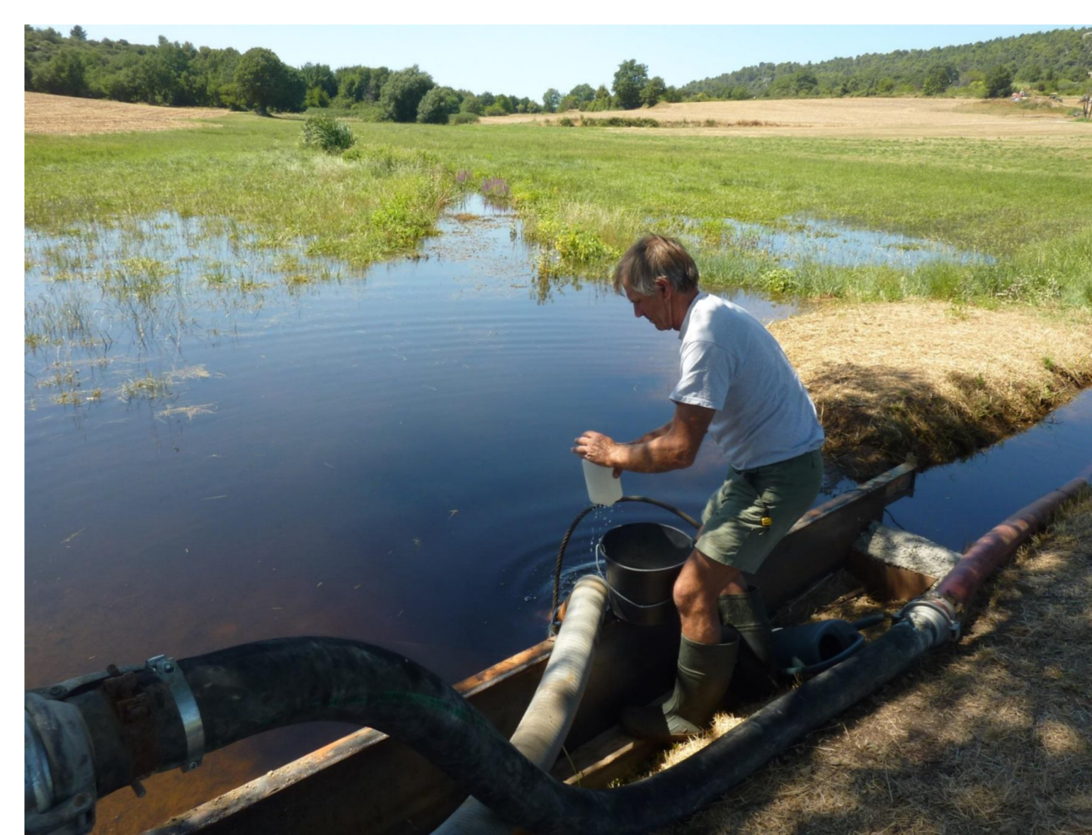
Setting up a storage – lagooning pond for an irrigation test 1 000 m 3 temporary pond and 50 m 3 /h pumping system
